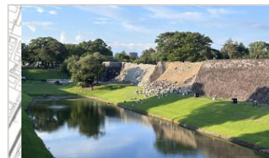
No.16西出丸石垣 崩落
